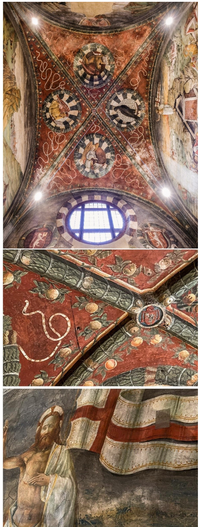
Figure 3. Intrados of the vault of the Castiglioni Chapel and evident deterioration and criticalities of the wall frescoes.
