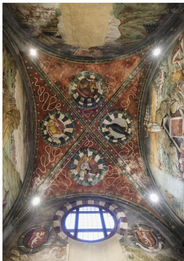
Fig. 1 Intrados of the vault of the Castiglioni Chapel and evident deterioration of the wall frescoes.
