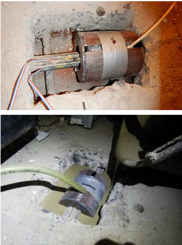
Fig. 2. The fully equipped ME sensor installed on the prestressed cable in the inspected bridge (above) and consequent filling of the created opening by the special grout (below)
