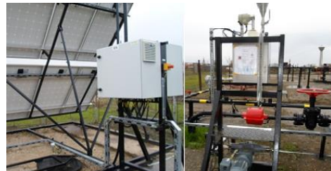
Fig. 5. Control and Chemical Dosing Equipment
