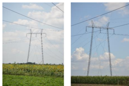
Figure 1. The towers on the analyzed span of the 220 kV overhead power line.
