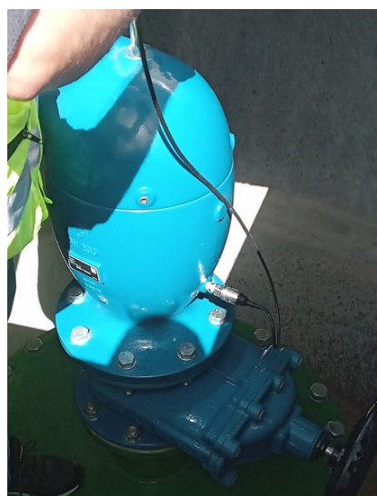
Figure 4. Pressure transducer connected to one of the pipe's air valve plug.
