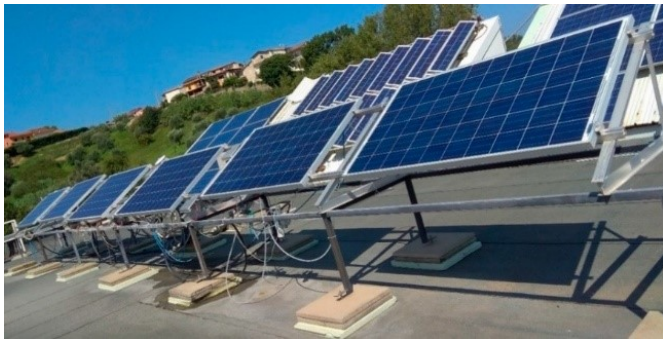
Figure 1. Experimental plant located at the cube 45C of the Department of Mechanical, Energy and Management Engineering of the University of Calabria.
