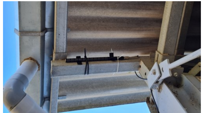
Figure 9. Installation of the microphone with clamps under the eaves of the barn to remain sheltered from the weather.
