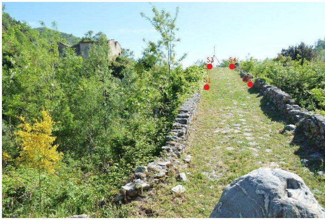
Figure 13. The positioning of the POIS 2.0 sensors on the extrados of the bridge.
