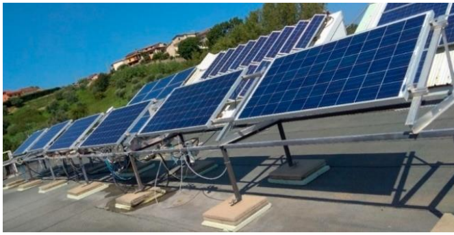
Figure 1. Experimental plant located at the cube 45C of the Department of Mechanical, Energy and Management Engineering of the University of Calabria.
